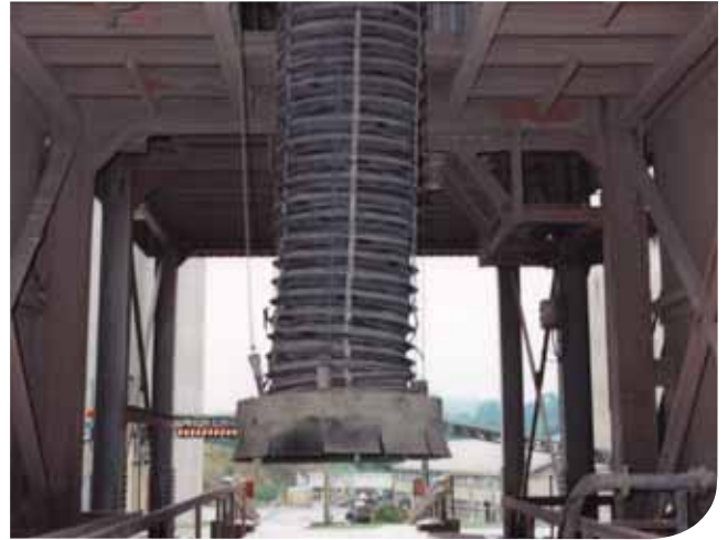
A wire reinforced bellow used to control the flow of powdered cement during loading
